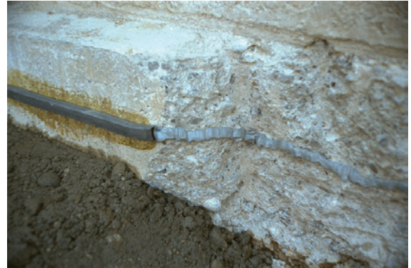
Rough Concrete Cold Joint
